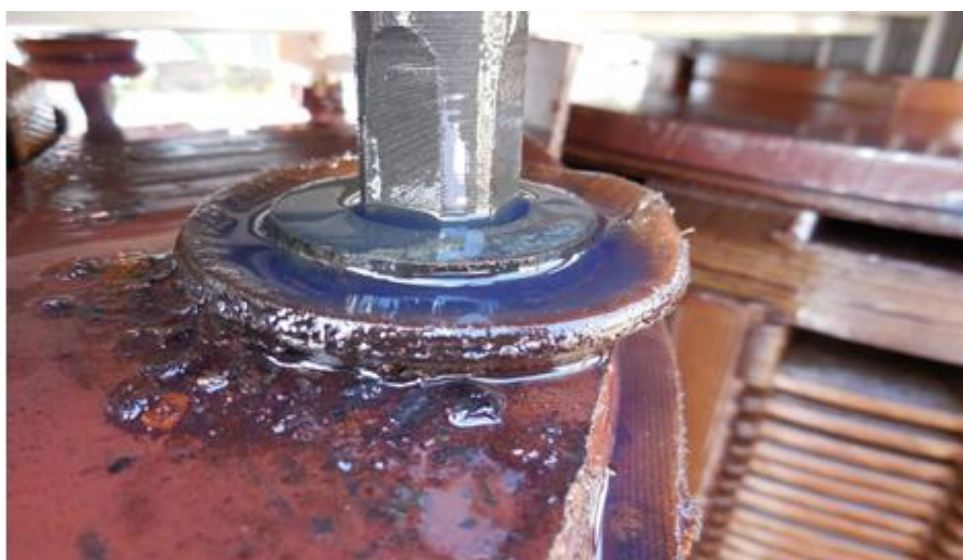
Fig. 1. Defect of the TM-1000/35 transformer, discovered during its opening.
